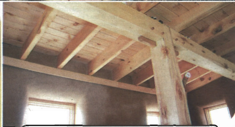
(above) Clay plaster smoothed over the straw and framing covers the interior walls with a design element similar to adobe.
